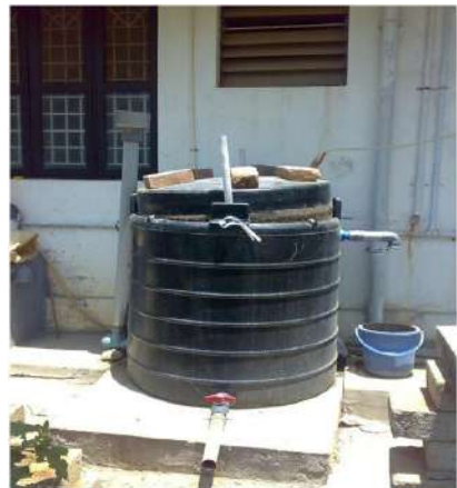
Kitchen waste Biogas Plant
