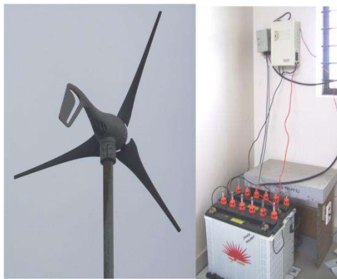
Wind-solar Hybrid system
