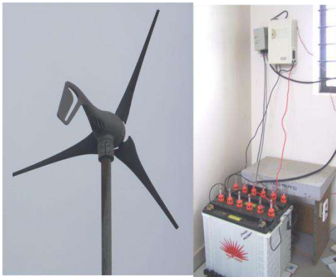
Wind-solar Hybrid system
