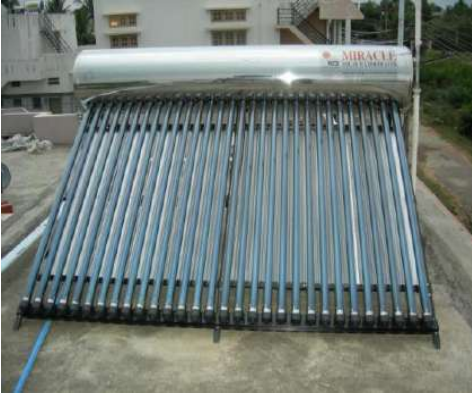
Evacuated Solar Water heater
