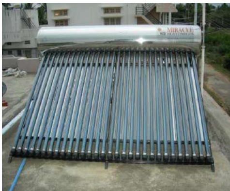
Evacuated Solar Water heater
